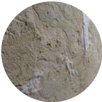
Spalling and salt efflorescences; high salt pressure
